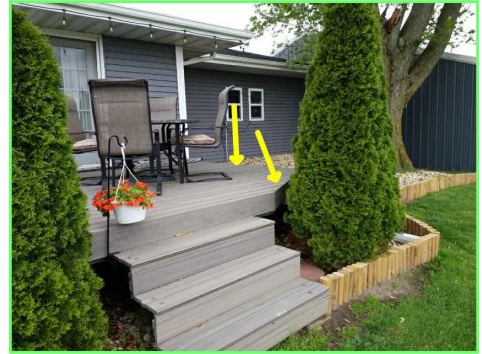
No Railing Present
