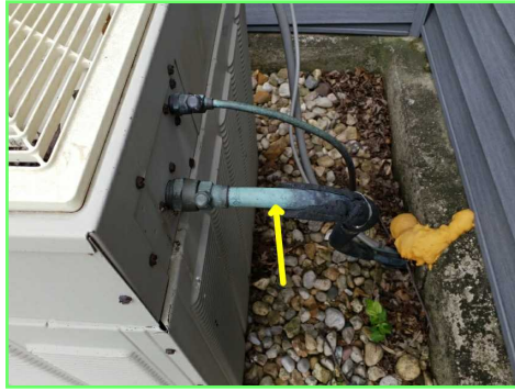
Damaged Insulation on Refrigerant Line
