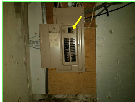
Electrical Main Disconnect
