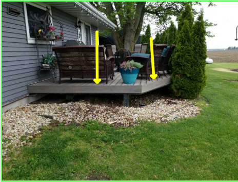
No Railing Present
