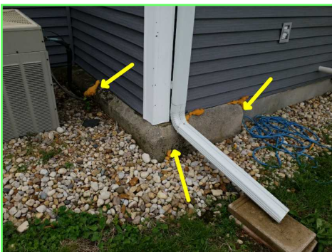
Cracks In Foundation
