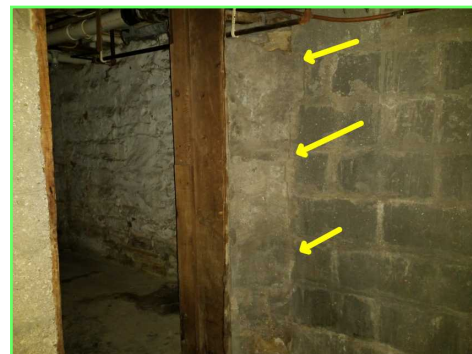
Cracks In Foundation
