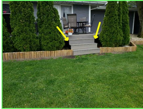
No Handrail Present
