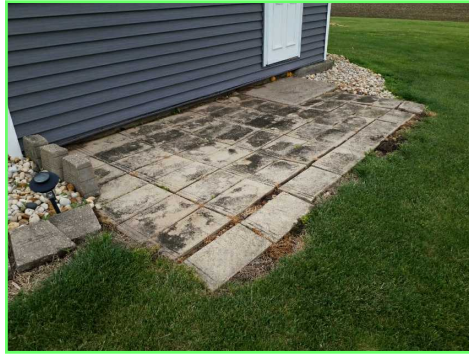
Blocks Have Settled
