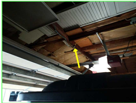
No Junction Box Present
