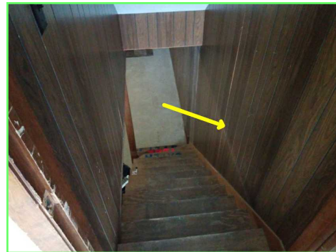
No Handrail Present
