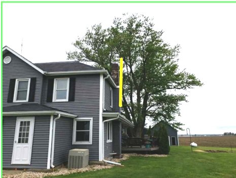
Chimney Is Out Of Plumb
