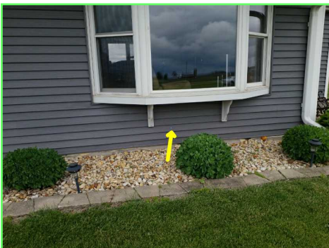
Hole in Siding
