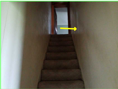
No Handrail Present
