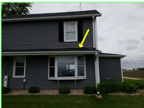
Flashing Pulled Away
