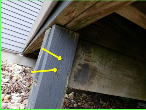
Post are Not Properly Secured
