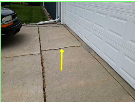
Cracking In Driveway
