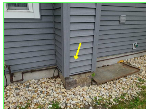
Hole in Siding
