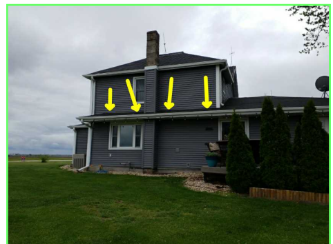
Flashing Pulled Away
