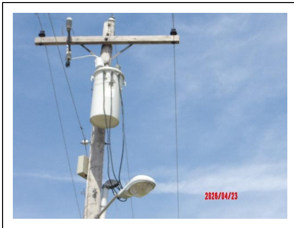
Transformer at Pole
